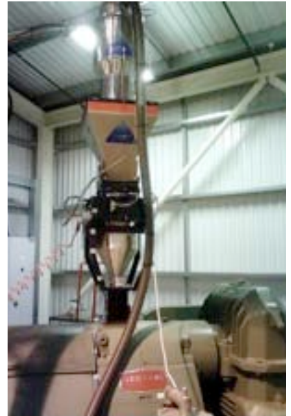
LIW Installed at Prysmian
